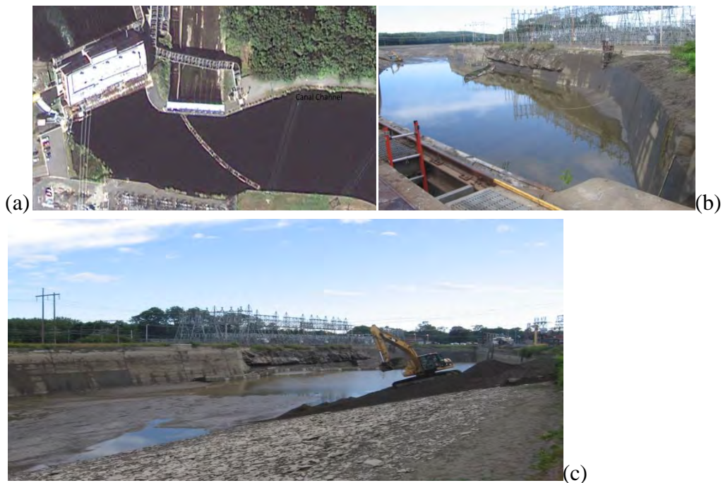
Location of Zone 1 (a) and typical views of Zone 1 during the drawdown (b and c).
