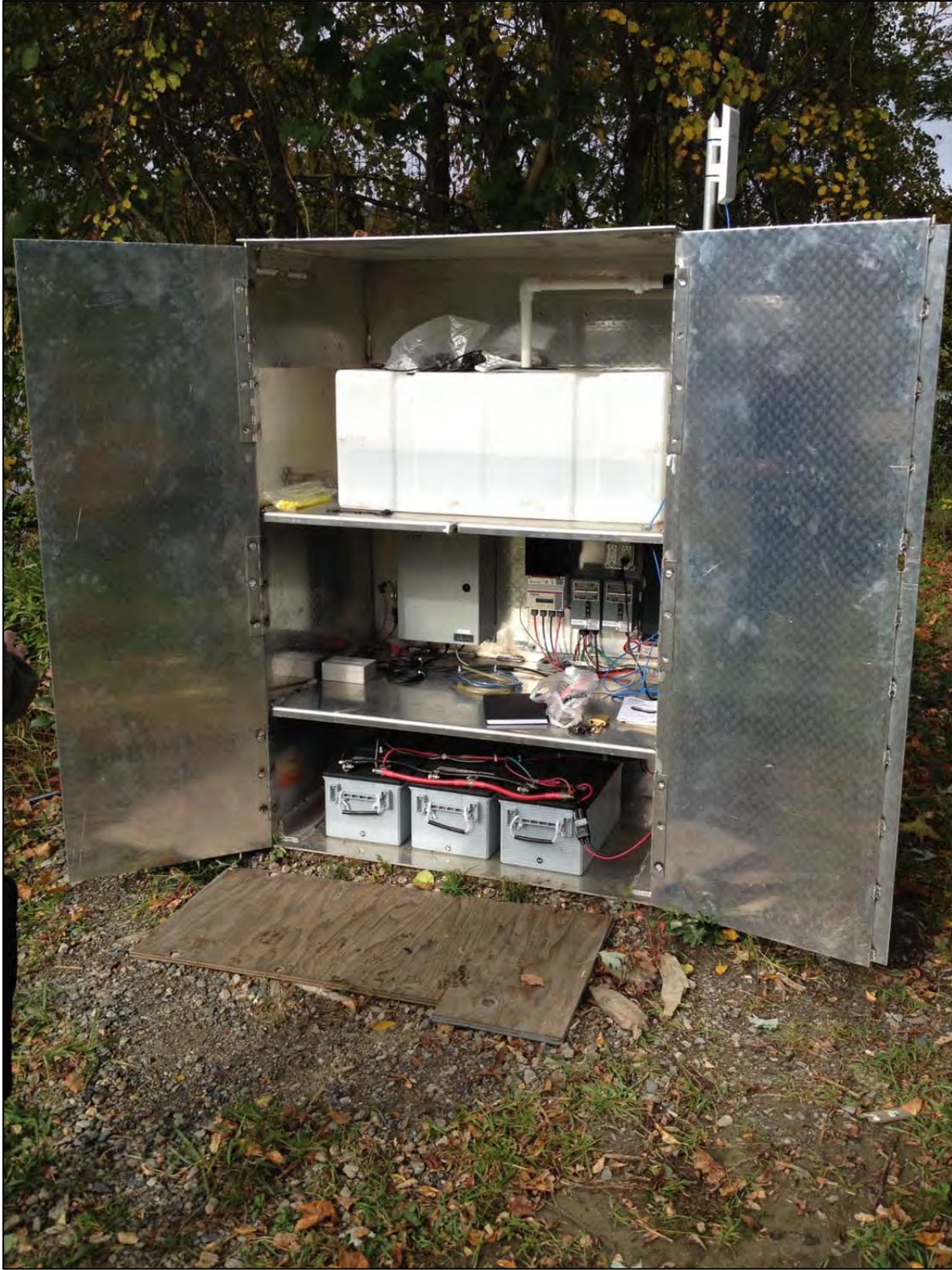
Figure 3.3: Typical configuration of LISST HYDRO as installed at the Northfield Mountain Tailrace (North HYDRO shown). Batteries for each instrument were charged using solar panels.
