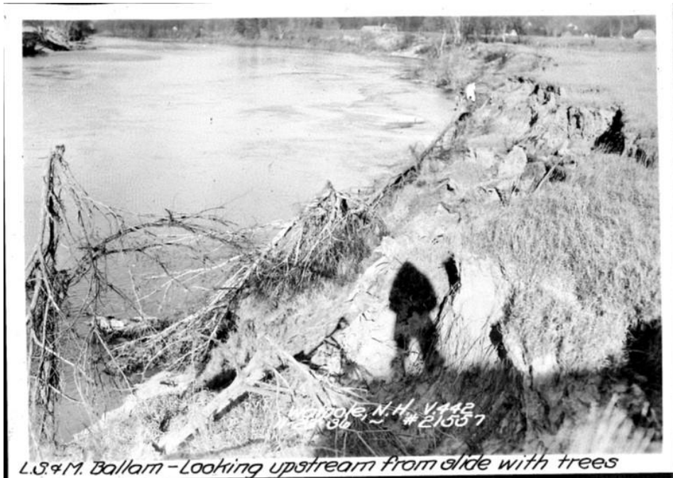
Figure 5.5.5.5-1 Erosion Damage – 1936 Flood
