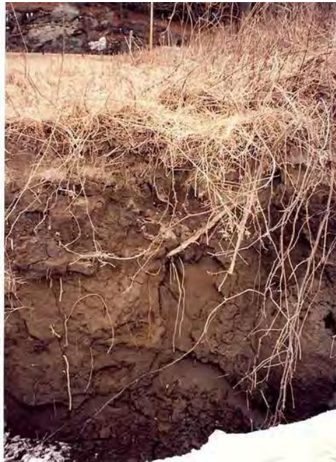
Figure 5.5.5.3-2 Cracks in a Riverbank Potentially Associated with Freeze-Thaw
