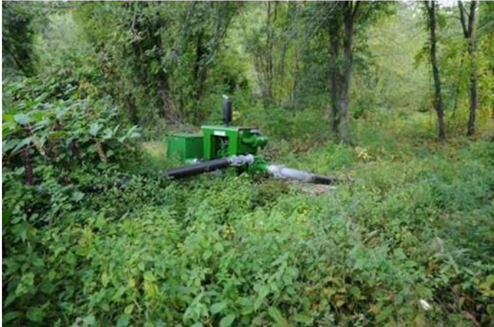
Figure 5.5.4-6a: Irrigation pumping from the Connecticut River, Photo 359
