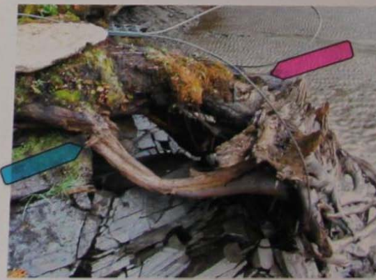
Summer 2012 - Root Stump Erosion, hemlock tree gone On the "Horse Race" - Montague MA
