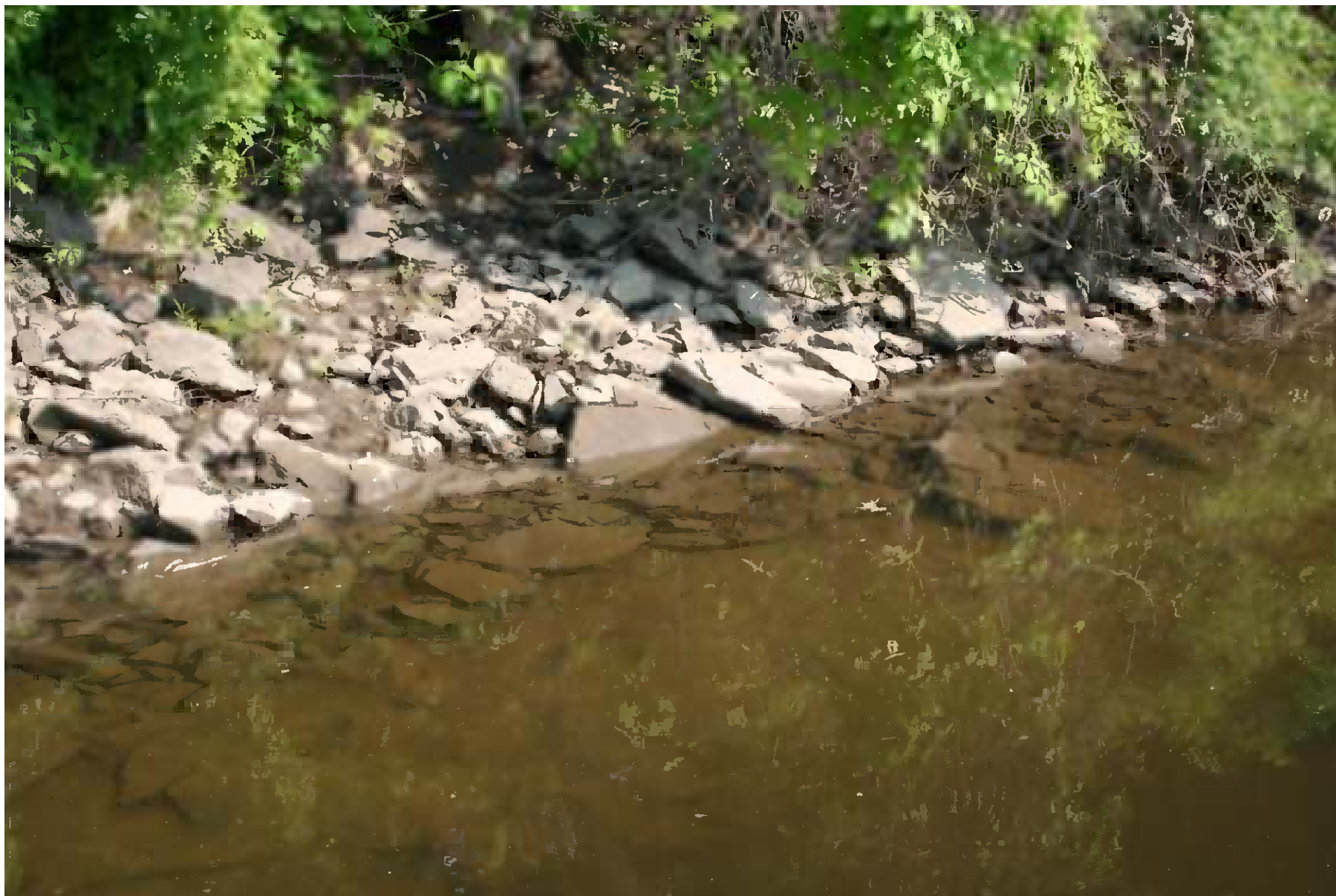
Figure 36: Notching above rock armoring with resulting minor erosion across from the Northfield Mountain Pumped Storage Project tailrace.
