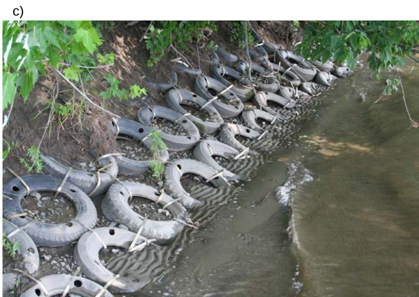
Figure 37: Experimental bank protection efforts using a) concrete mattress, b) tire wall, and c) tire mattress downstream of Route 10 Bridge.
