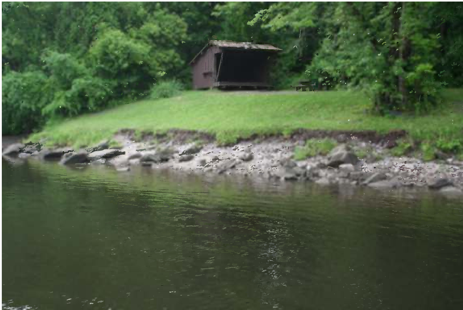
Figure 35: Failing rock armor at Munn's Ferry picnic area.
